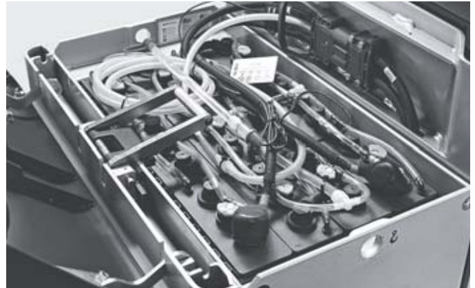
Ultimate availability: either with lateral lead-acid battery changing as standard, for fast, safe replacement, or with interim charging of a lithium-ion battery
